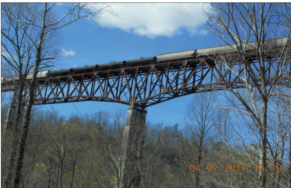
Left: Norfolk Southern's New River bridge, 389 feet above the river in Tennessee
